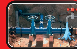
Water Pipe Line
